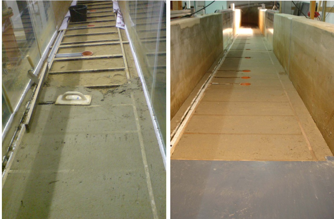
(a) Downstream view of the beach wedge and the installation of the floating screed (b) PVC board, the finished floating screen and the cable duct for the pressure sensor connections
